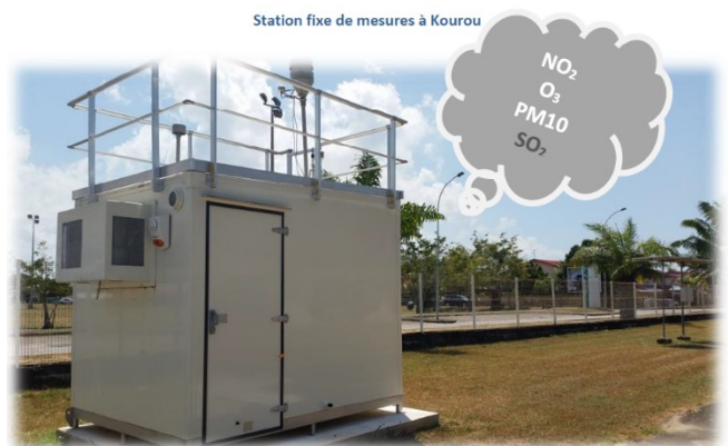
Figure 7 : Station de surveillance BRADY à Kourou, ORA 2016
